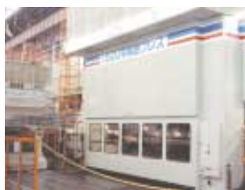
Installed sound-insulating box for stamping machinery (double structure)
