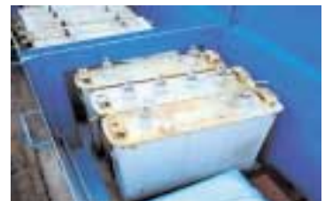
PCB-containing condensers in storage
